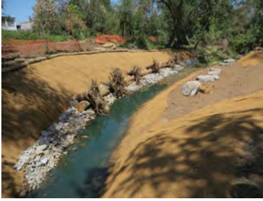
Arcade Creek Park and Preserve - Project site after biotechnical bank stabilization techniques applied.
